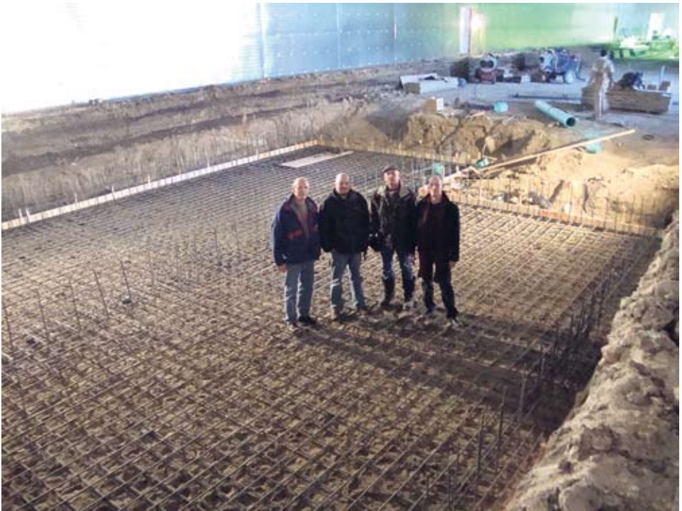
L-R Daniel Stechey (Canadian Aquaculture Systems Inc), Greg Beckman (Water Management Technologies Inc.), Rudy Reimer and Jeff Eastman (MB Agriculture Food and Rural Initiatives) oversee construction of the first Canadian Model Aqua-Farm at the Reimer’s farm in Warren, Manitoba.
